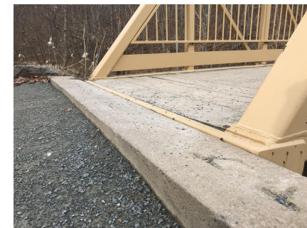
Miner's Marsh, Bridge - Grading Required
