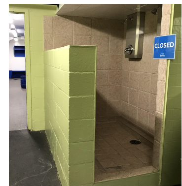
Centennial Arena, No Accessible Showers
