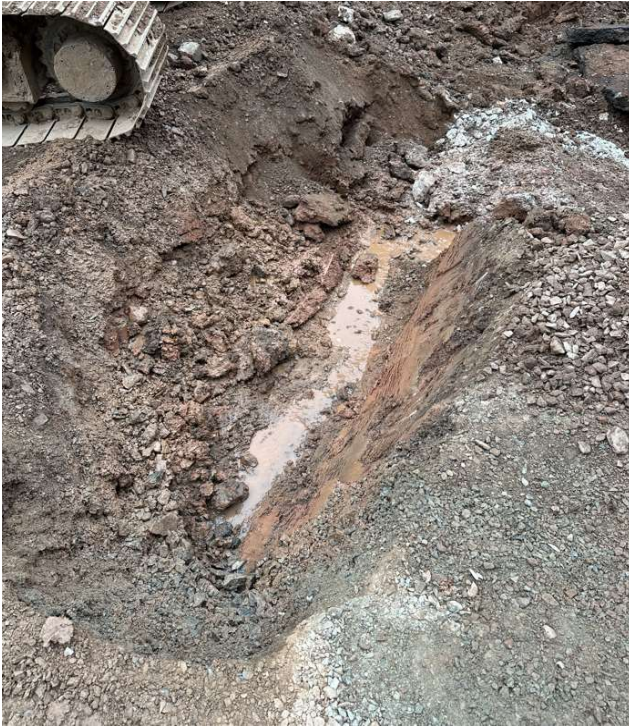
Water flowing from clear storm at Civic #399. GPEL removed lateral.
