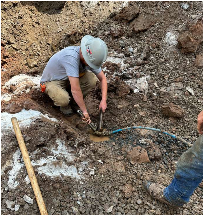
Water main at Civic #420/422 broken and repaired.
