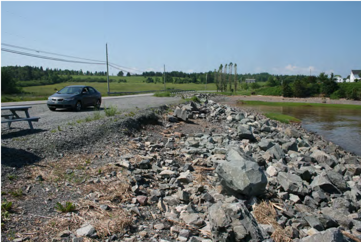
Cheverie Bridge (Stop 10). Inadequate armouring allows overtopping by waves that continues to erode the shoulder of Highway 215. Photo: Philip Finck
