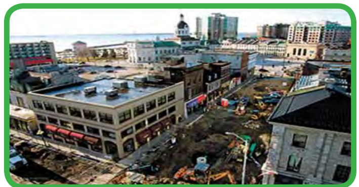
Major efforts to replace older infrastructure in downtown Kingston has facilitated new growth opportunities.
